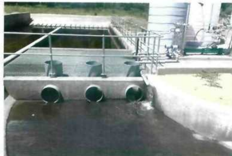
Clean water discharge after the installation of Ultraspin at coal mine.
