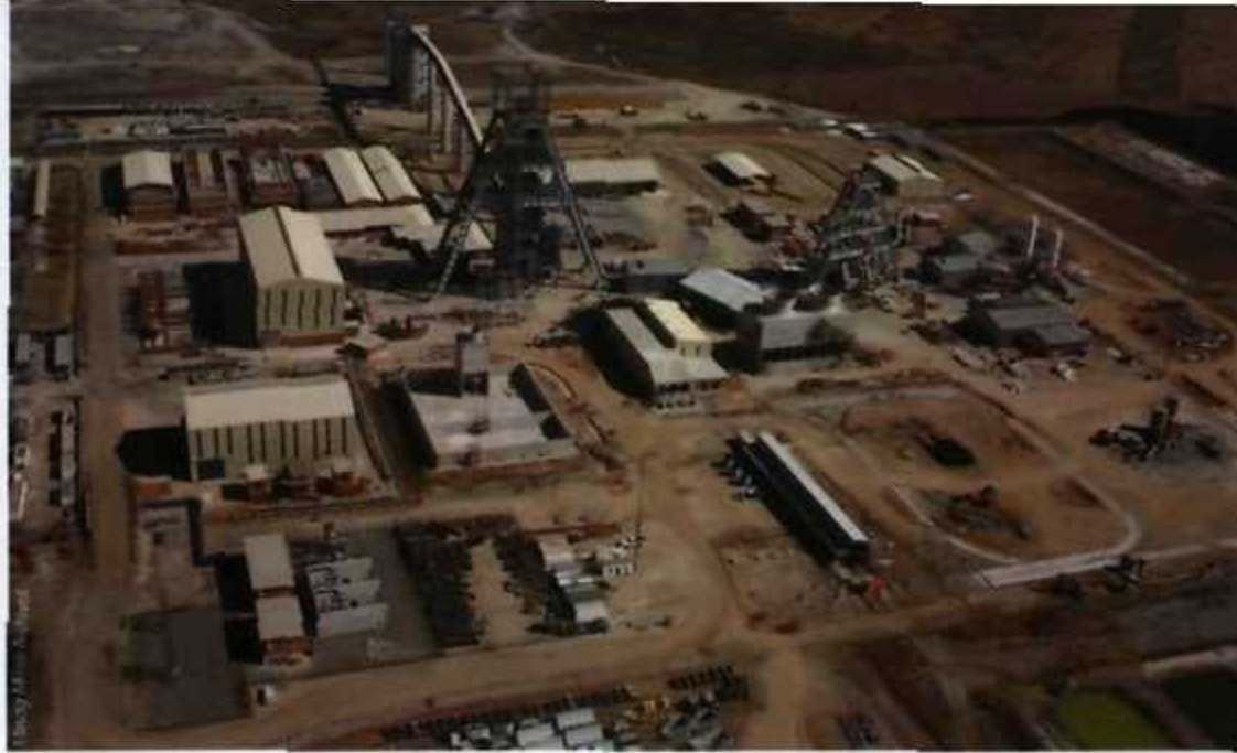
Steel offers the faster method of construction when it comes to headgear.
