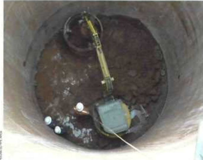
ZERO SWING The R35-7Z allows for performance close to walls and obstacles without damaging the machine
