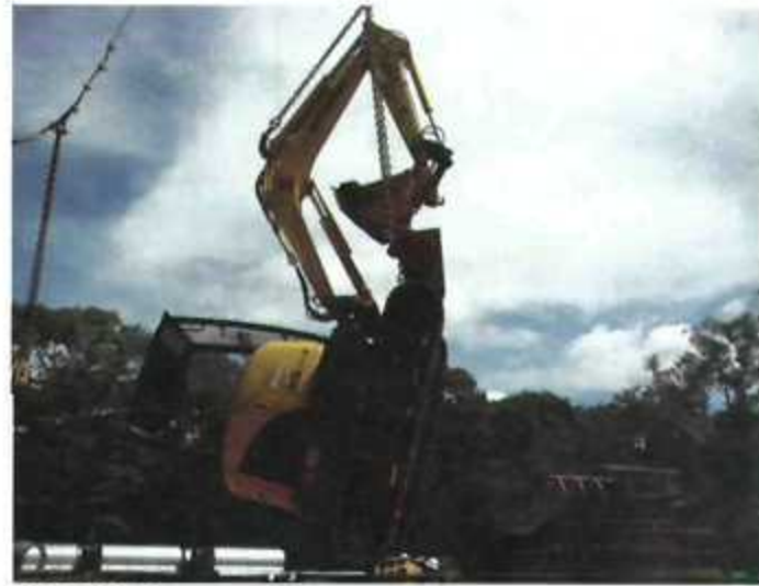
HEAVY WORK The 3,5-t machine is lowered into the shaft up to five times a day
